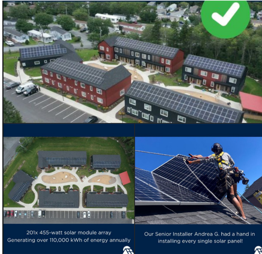
Photo by Solar Ascent
