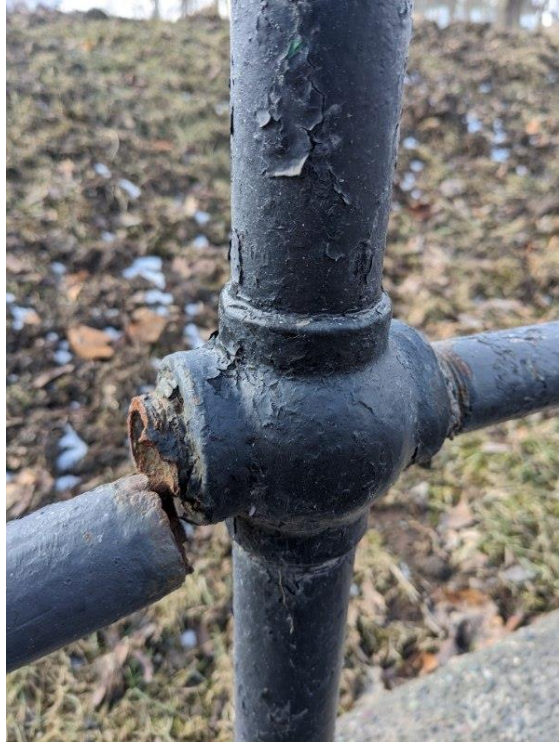
Figure 4 – Sheared Connection Between Horizontal rail and Vertical Post
