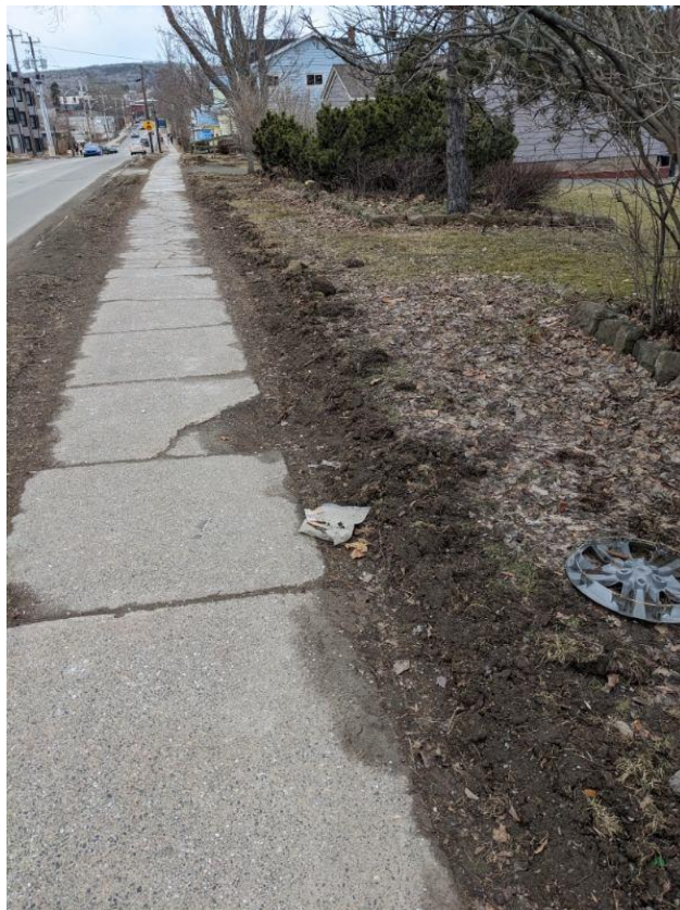
Figure 5 – Evidence of Surface Disturbance on Town Right-of-Way Near Handrail Location
