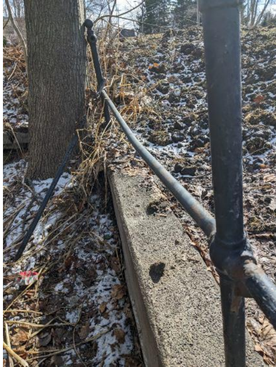
Figure 2 – Inward Deflection of Horizontal Handrail Toward 91 Church Street Property
