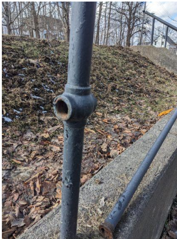
Figure 3 – Sheared Connection Between Horizontal rail and Vertical Post
