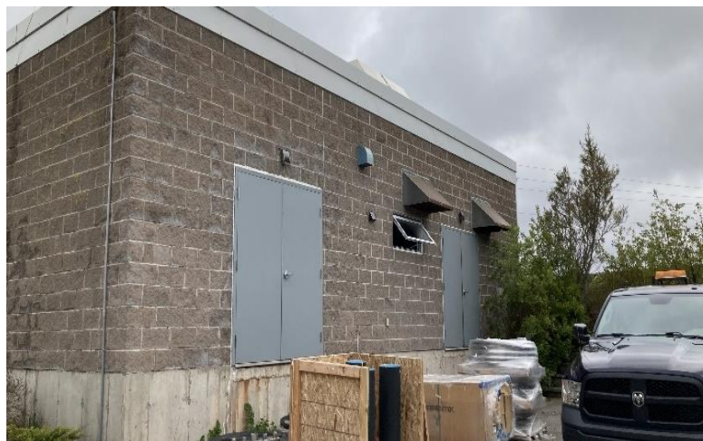
Figure 7.1: Antigonish Wastewater Plant
