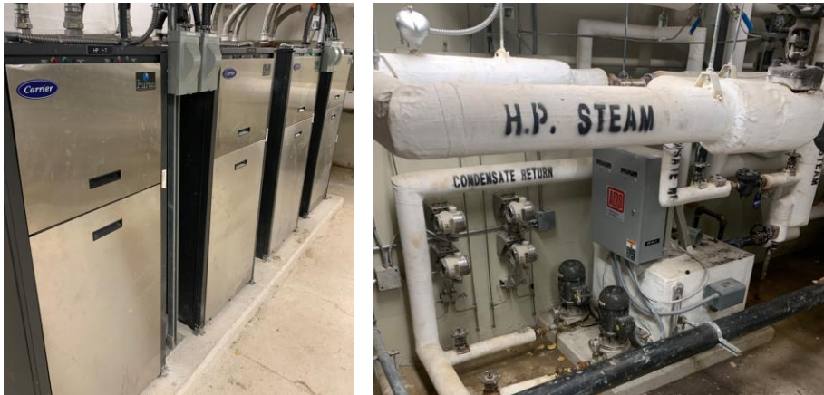
Figure 1: Central water to water HP units & steam PRV – Schwartz
