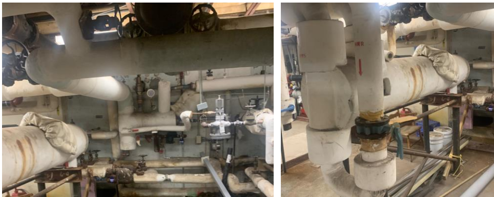
Figure 2: Main steam entrance & steam heat exchanger (HX) – MacDonald Library
