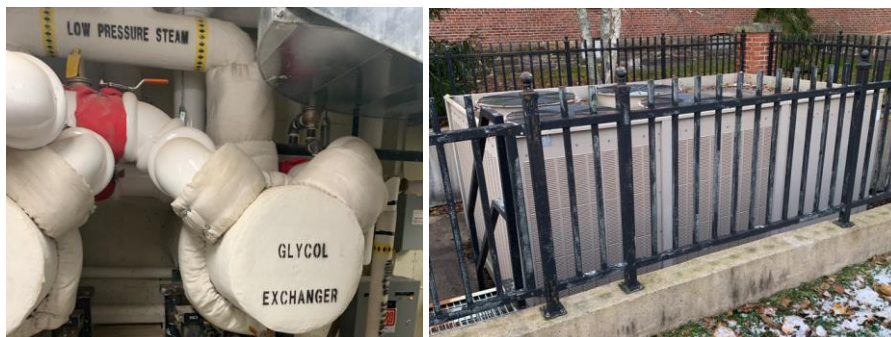
Figure 23: Glycol exchanger & Chiller - Coady (East)
