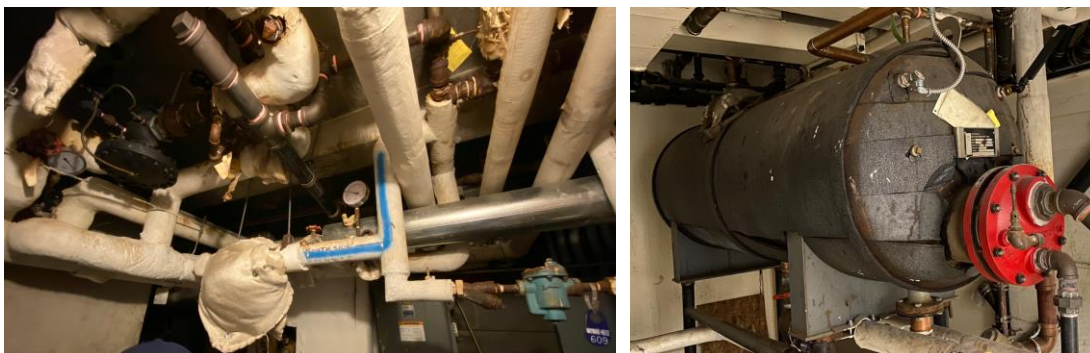
Figure 22: Main steam entrance & DHW tank - Cameron Hall
