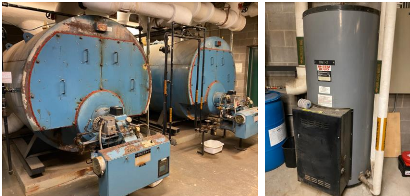
Figure 29: Boilers & a DHW unit - St. Andrew Junior High
