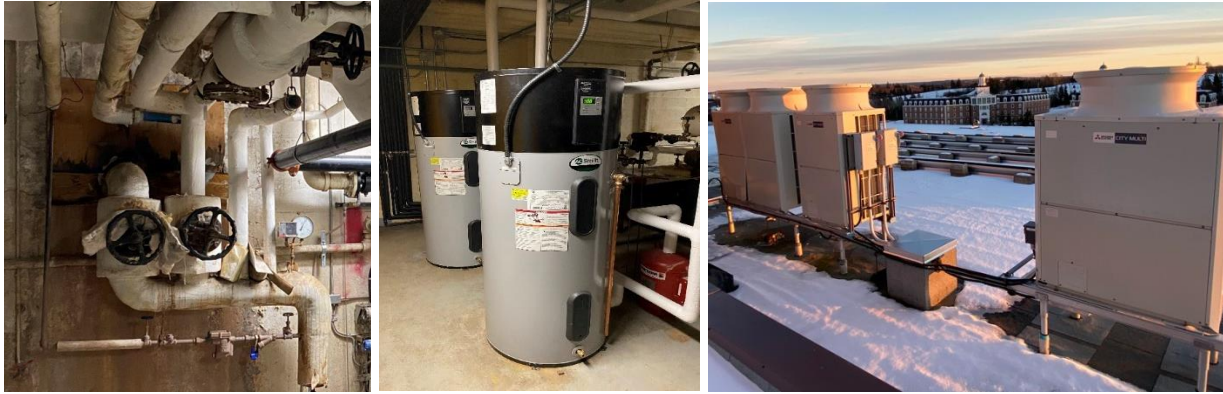
Figure 9: Main steam entrance, DHW & VRF units - Bloomfield Centre
