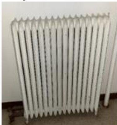
Figure 4: Hot water baseboard – Camden Hall
