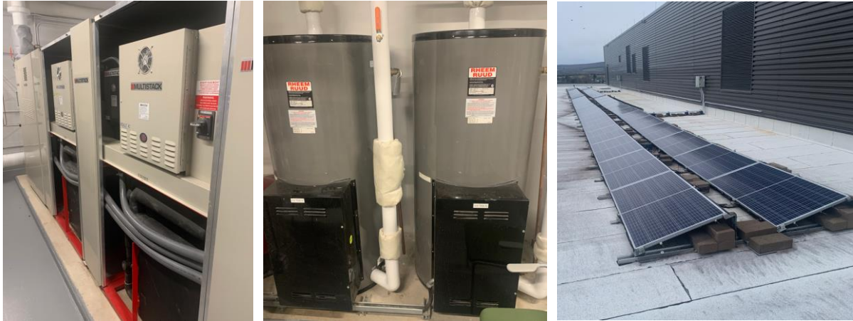
Figure 26: HP modules, DHW & rooftop solar - Mulrone Hall
