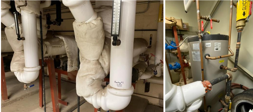
Figure 12: Steam HX – Keating Centre
