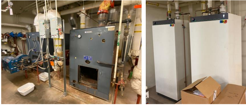
Figure 28: Boilers & Outdoor condensing units - Dr. John Hugh Gillis Regional High School
