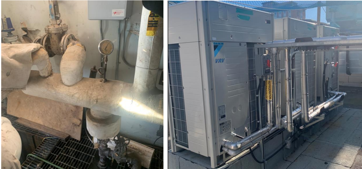
Figure 20: Main steam entrance & VRF units - Morisson Hall
