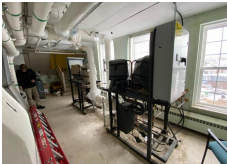
Figure 5: Chillers - Marguerite Hall
