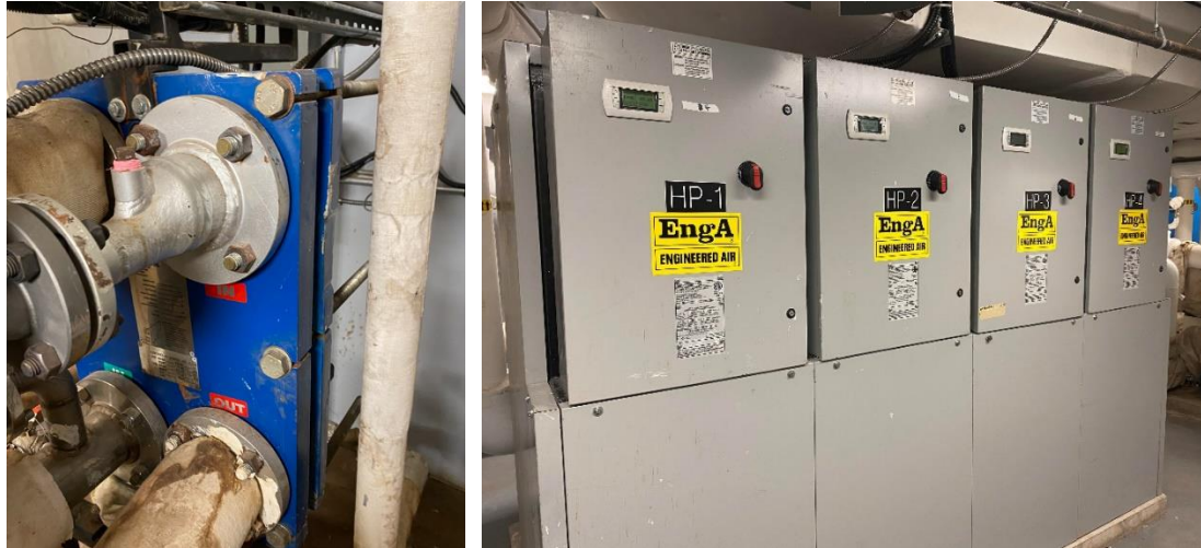
Figure 25: Steam to Glycol exchanger & HP modules - O'Regan & Riley Hall
