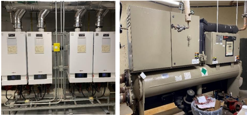
Figure 8: Propane Boilers & Chiller - JBB
