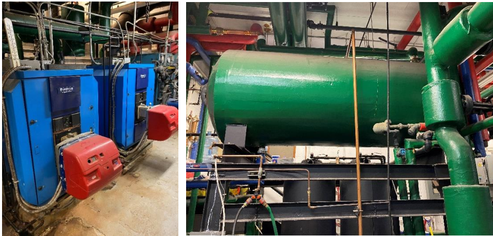
Figure 31: Boiler & Hot water tank - RK MacDonald Home
