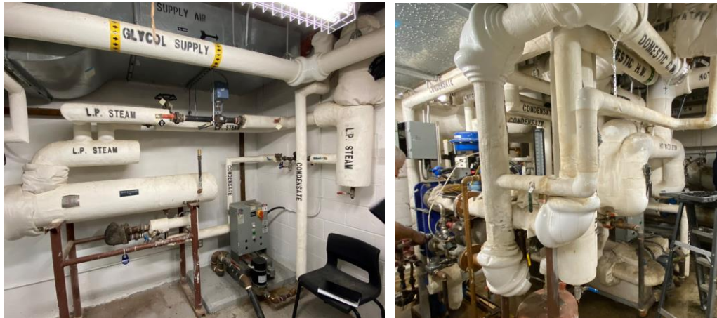
Figure 16: Main steam entrance & steam HX - Bishops Hall
