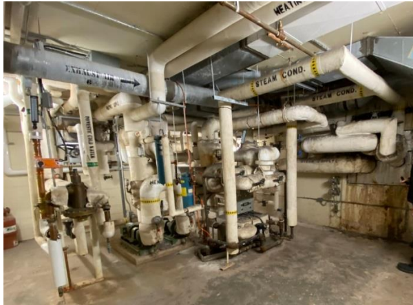
Figure 10: Main steam entrance & steam HX - MacIsaac Hall
