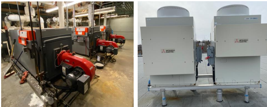
Figure 27: Boilers & Outdoor condensing units - Dr. John Hugh Gillis Regional High School
