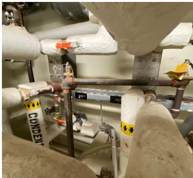
Figure 24: Glycol exchangers - Coady (West)
