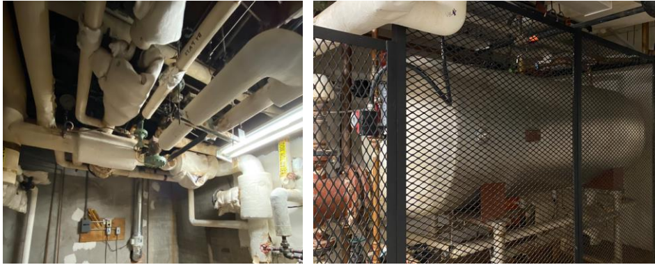
Figure 21: Main steam entrance & DHW tank - MacKinnon Hall
